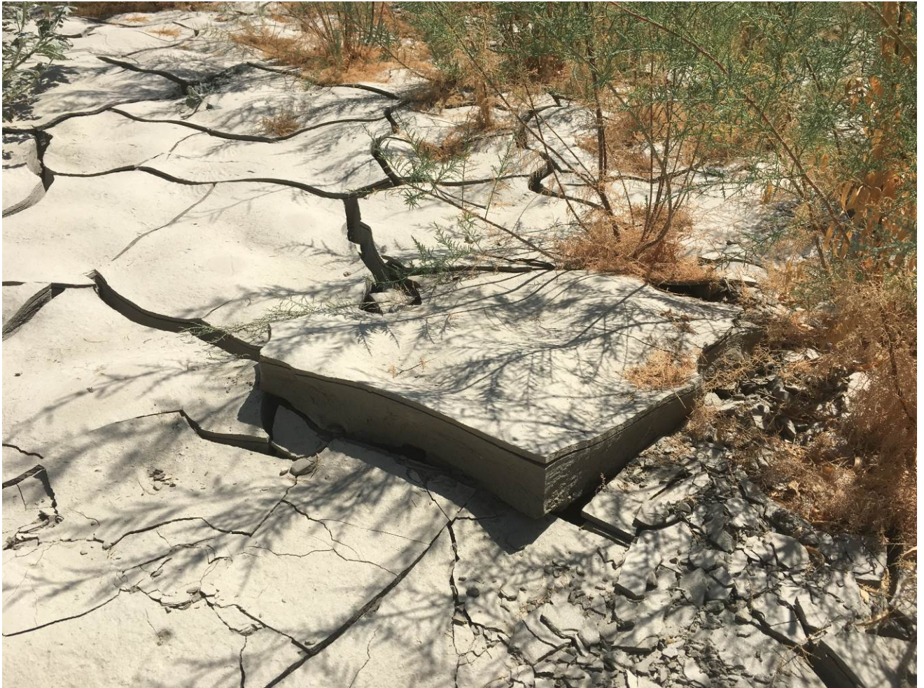
Photo 3. September 2017 accumulated silt in the pit
