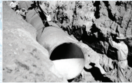
1953 - Installing the supply line under the bed of the San Jacinto River
