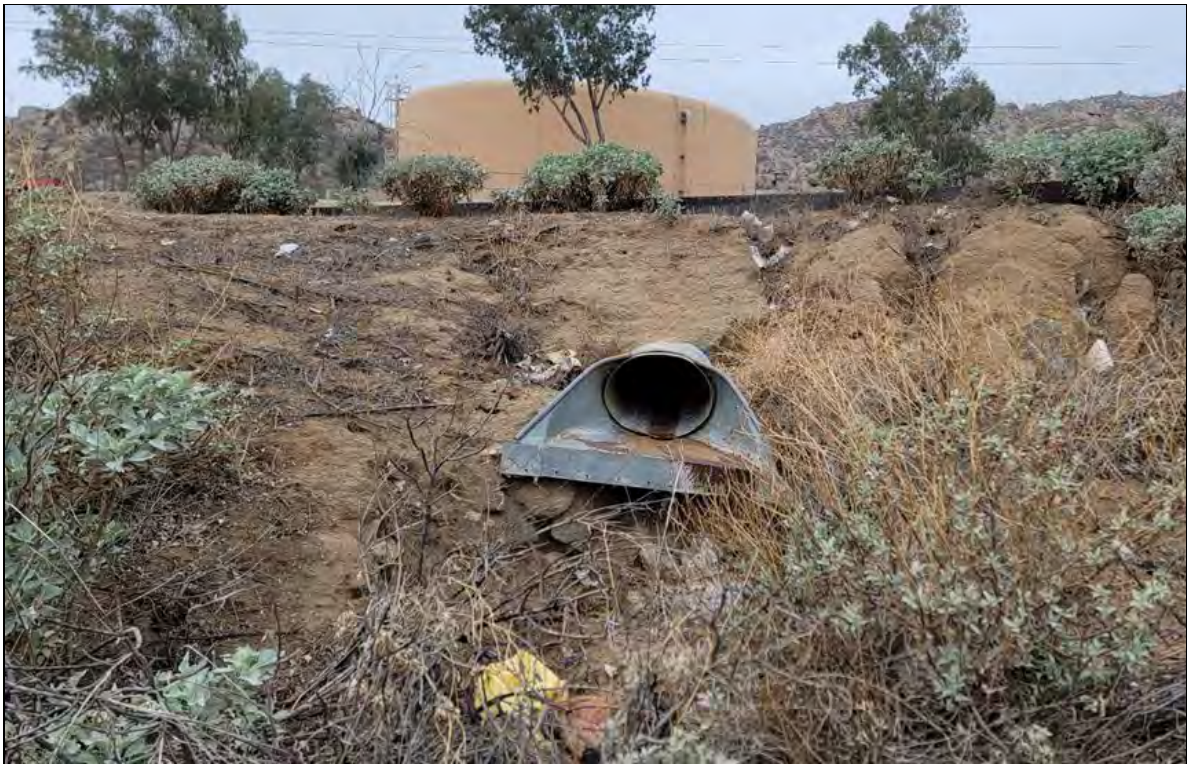
Photograph 17: View of eastern downstream 30-inch EF1 culvert on eastern side of Moreno Beach Drive, facing upstream and west. Culvert is proposed for complete removal, and an 18-inch storm drain to installed immediately north of this location.
