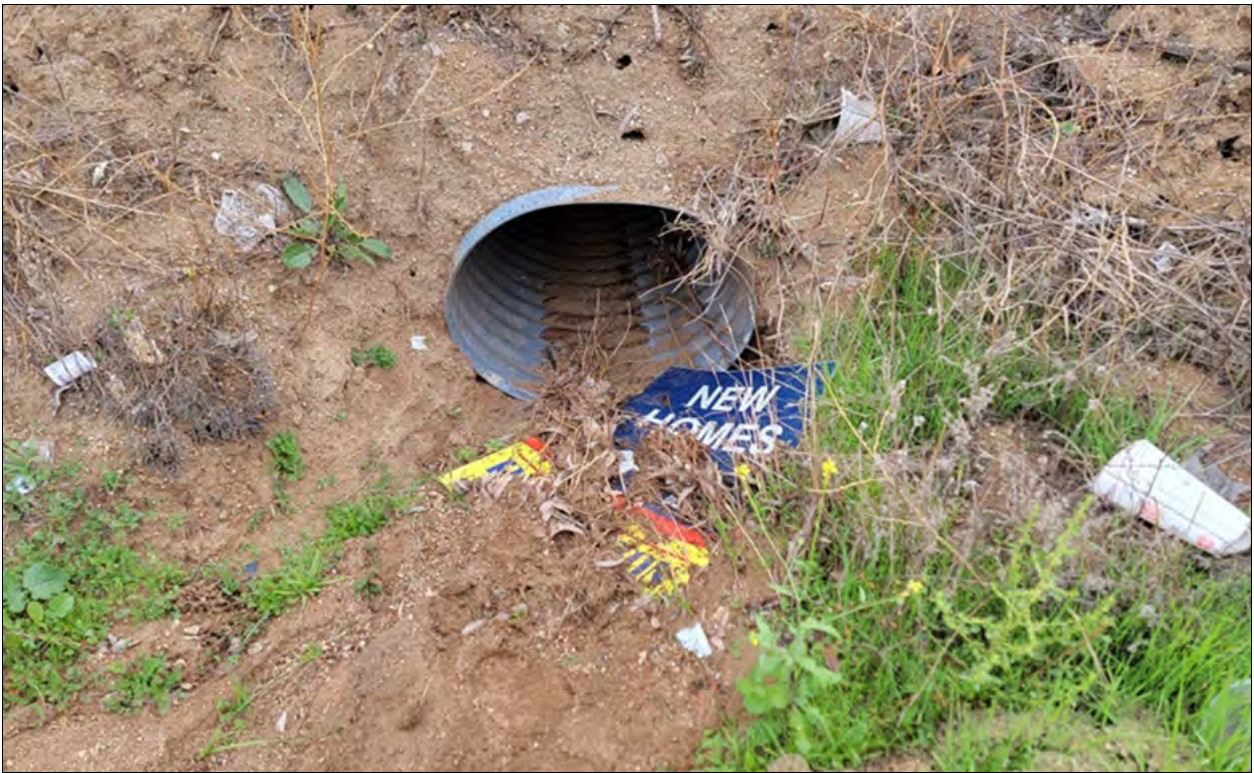
Photograph 7: View of western upstream inlet of 30" culvert for Drainage 1 on the western side of Moreno Beach Drive, facing downstream and east. Culvert is proposed for complete removal, and an 18-inch storm drain is proposed to be installed immediately north of this location.
