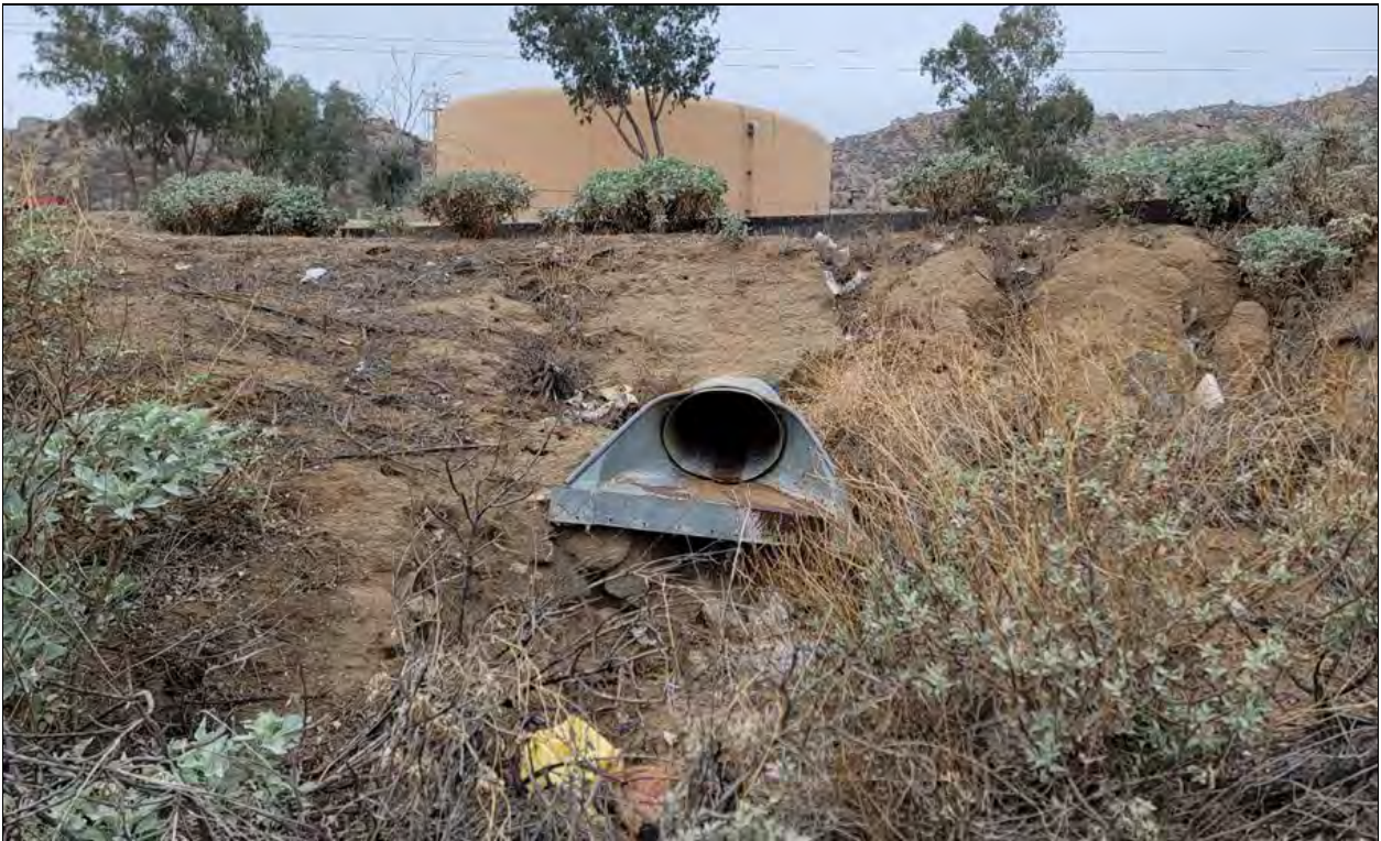
Photograph 9: View of eastern downstream 30-inch Drainage 1 culvert on eastern side of Moreno Beach Drive, facing upstream and west. Culvert is proposed for complete removal, and an 18-inch storm drain to installed immediately north of this location.
