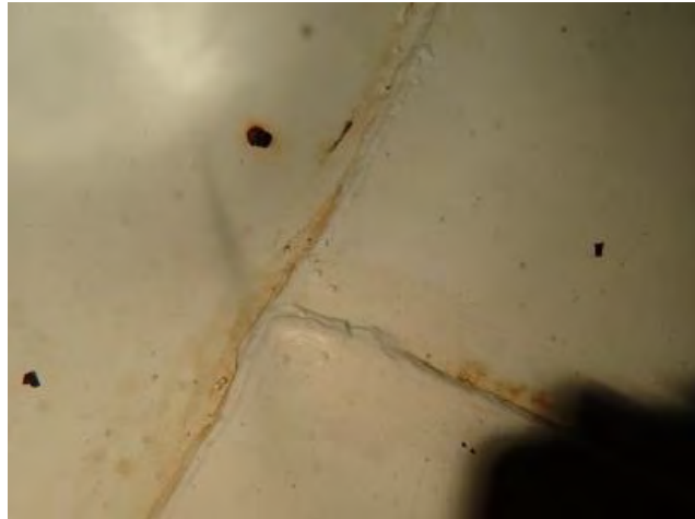
Figure 10: Floor plates with isolated corrosion spotting
