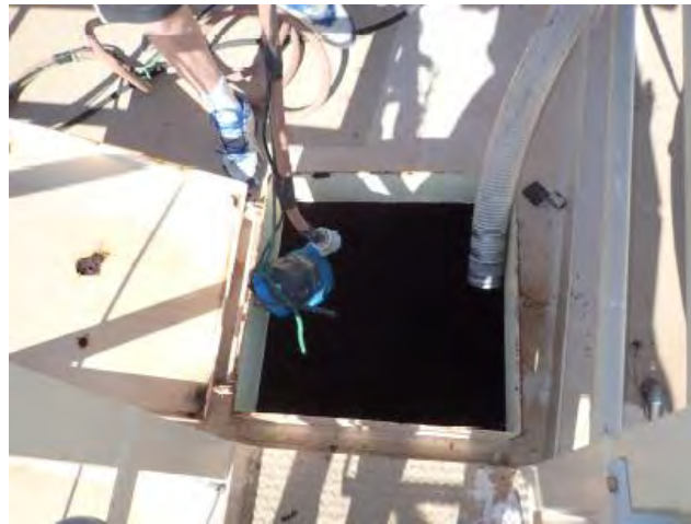
Figure 15: Roof hatch in moderate condition with areas of moderate corrosion
