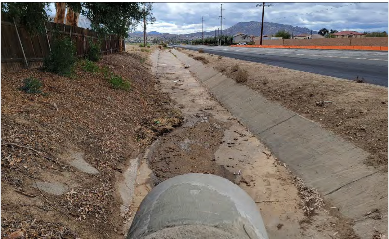
Photograph 14: View downstream of Drainage 4 from concrete culvert into 5-foot wide concrete lined channel portion, facing south along Moreno Beach Drive.
