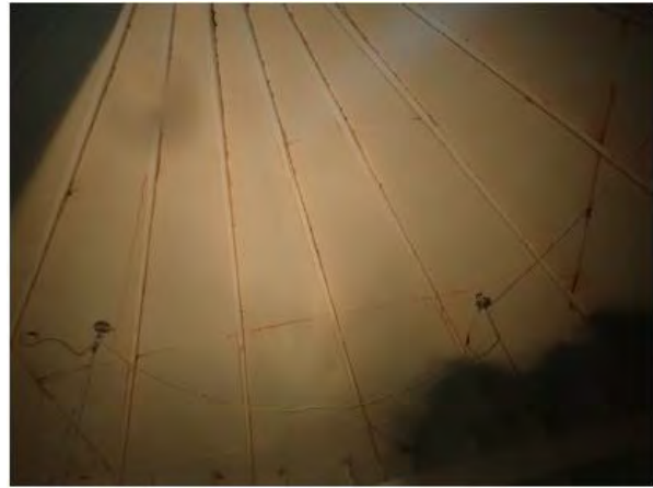
Figure 2: Moderate to minor corrosion along weld seams of roof plates
