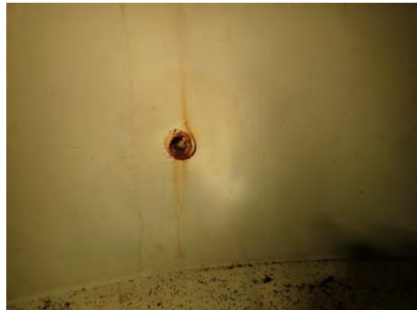
Figure 5: Penetration for level indicator with moderate to severe corrosion
