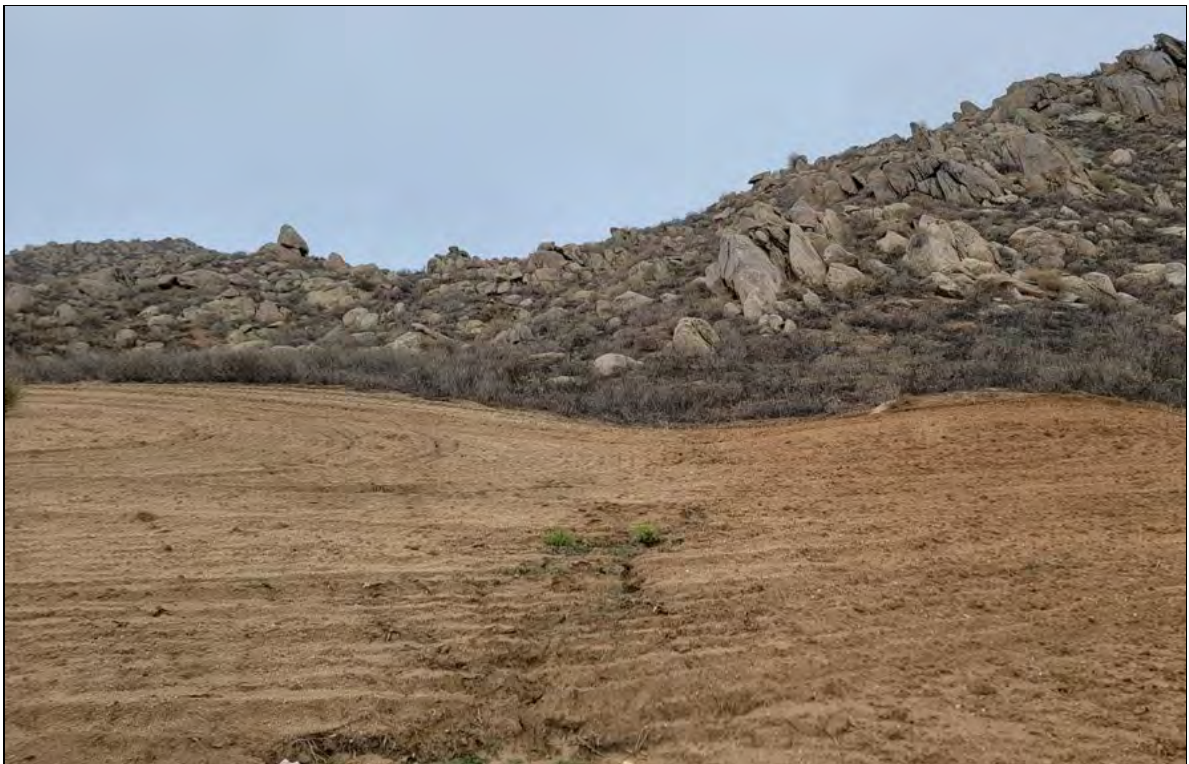
Photograph 14: View of erosional feature EF3 facing upstream and northwest from its intersection with Moreno Beach Drive.
