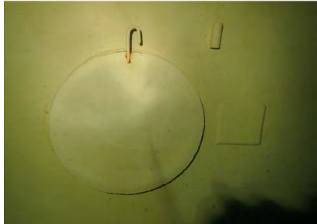
Figure 7: Man way entrance with minor rust on wing arm
