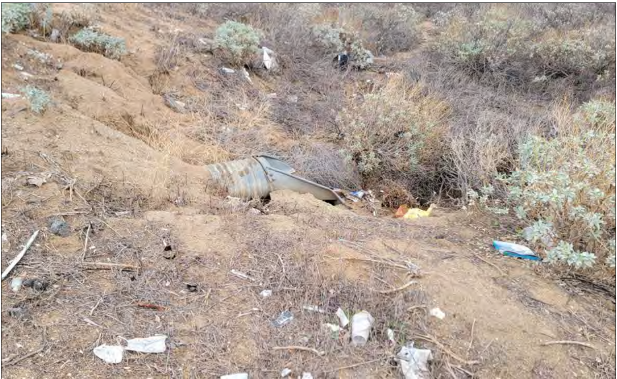
Photograph 8: View of eastern downstream outlet of Drainage 1 culvert, downstream and east of Moreno Beach Drive. Photo depicts existing 30" corrugated metal culvert which will be replaced with an appurtenant facility which includes an energy dissipater, headwall, rip-rap, 18-inch storm drain, and metal culvert.
