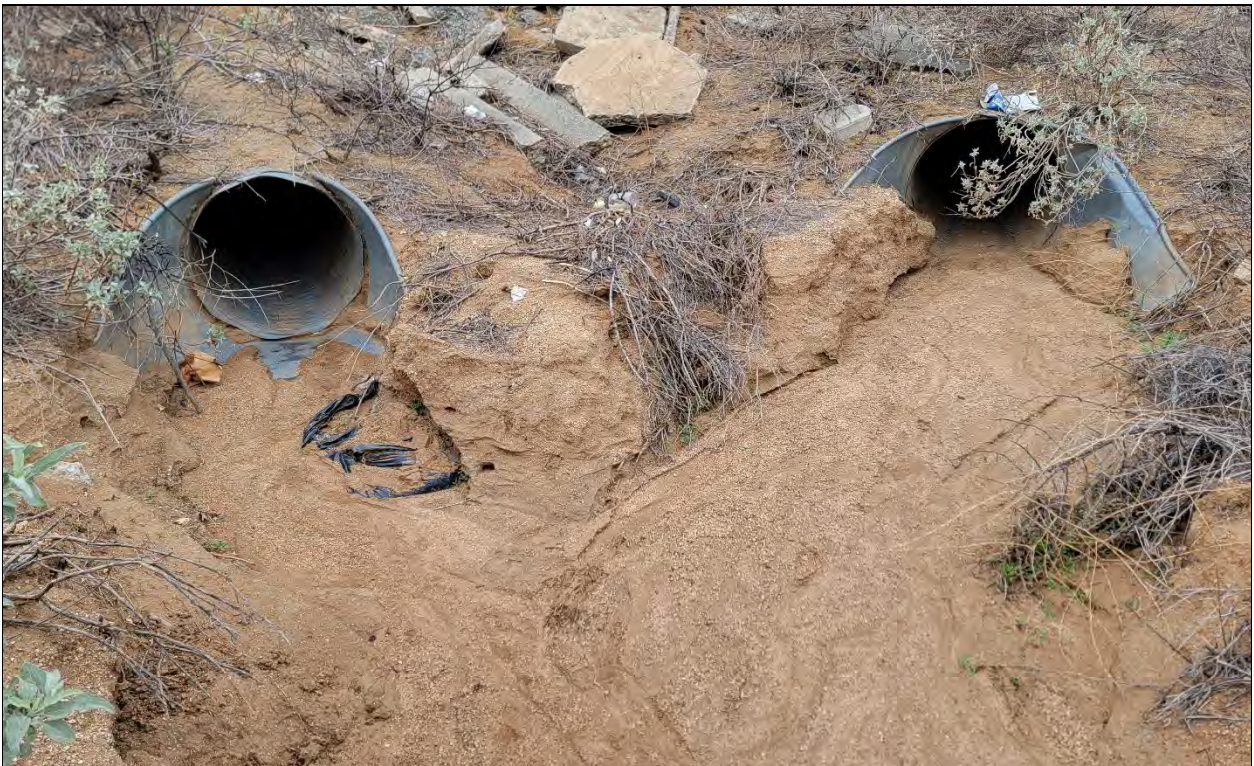
Photograph 12: View upstream towards two 30" culverts for Drainage 2 (left) and Drainage 3 (right), and their confluence just east of Moreno Beach Drive, facing west. Channel continues as a single drainage (Drainage 4) conveying flows to the east and southeast.
