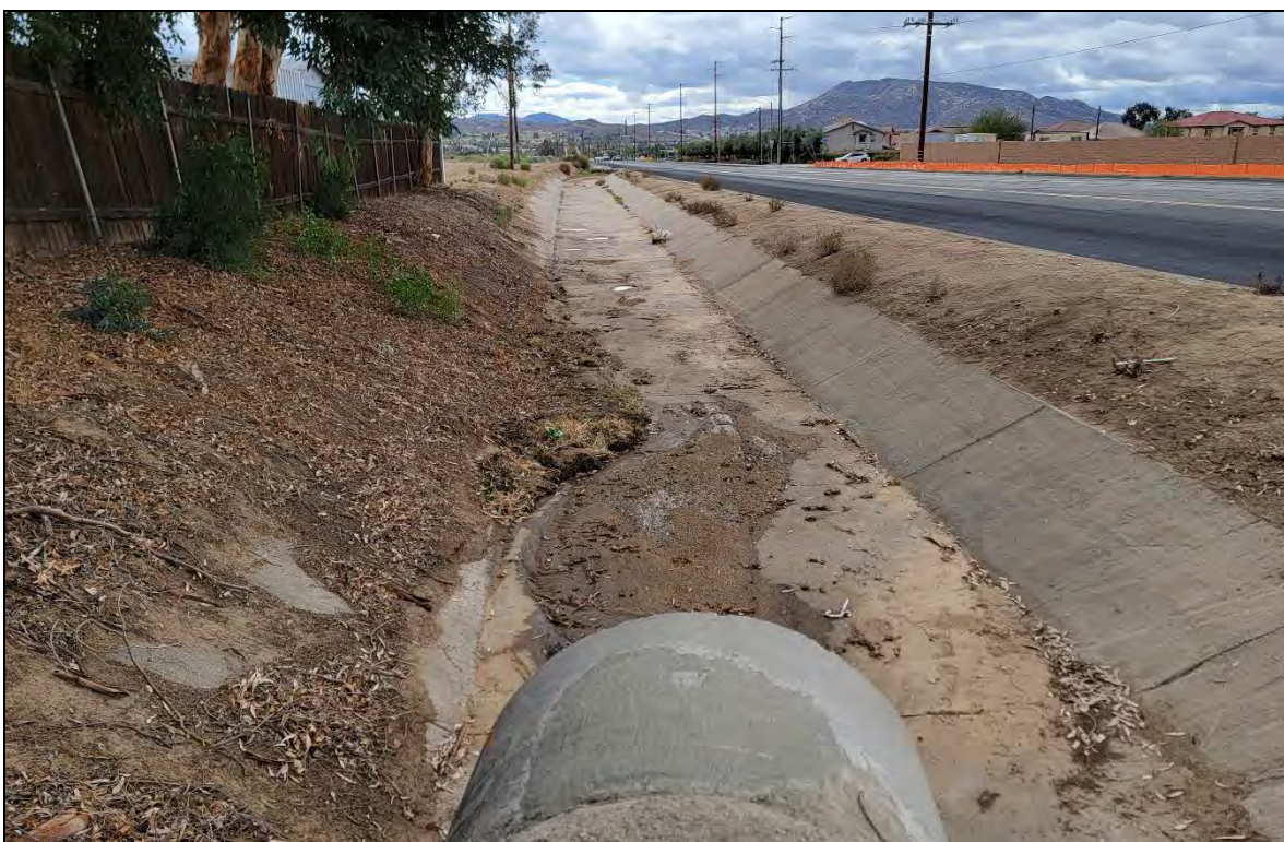
Photograph 22: View downstream from concrete culvert into 5-foot-wide concrete lined channel, facing south along Moreno Beach Drive.
