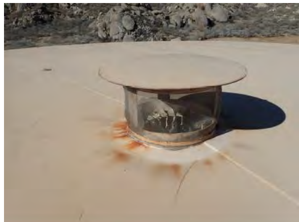
Figure 14: Roof vent in poor condition with moderate corrosion around base
