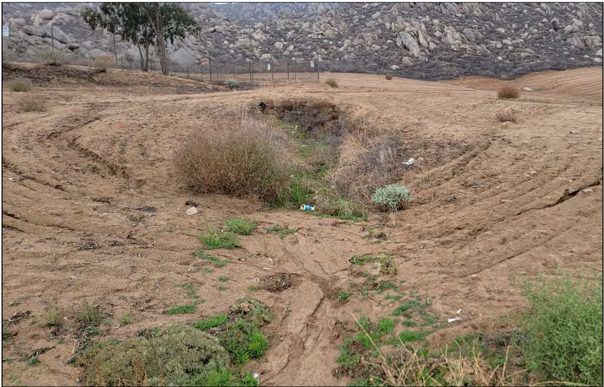
Photograph 9: View of erosional feature EF1, facing upstream and west from its intersection with Moreno Beach drive. Photo depicts the complete limits of EF1 within the grading limits, and its upstream boundary and metal culvert.
