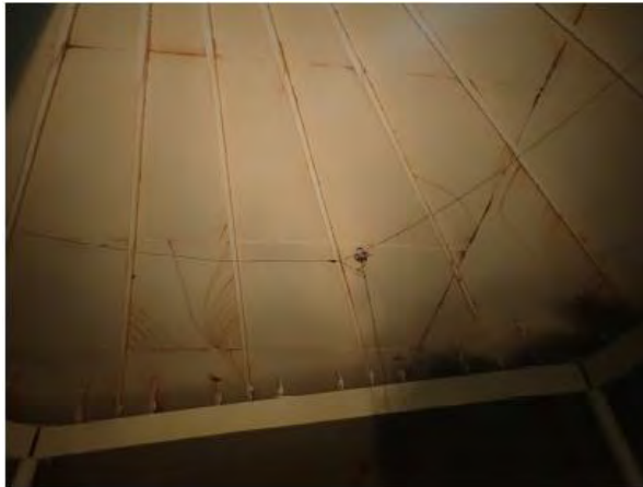
Figure 1: Moderate to minor corrosion where rafters meet kicker plates
