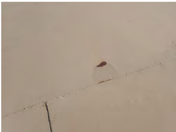
Figure 13: Roof plates in good condition with isolated corrosion spotting
