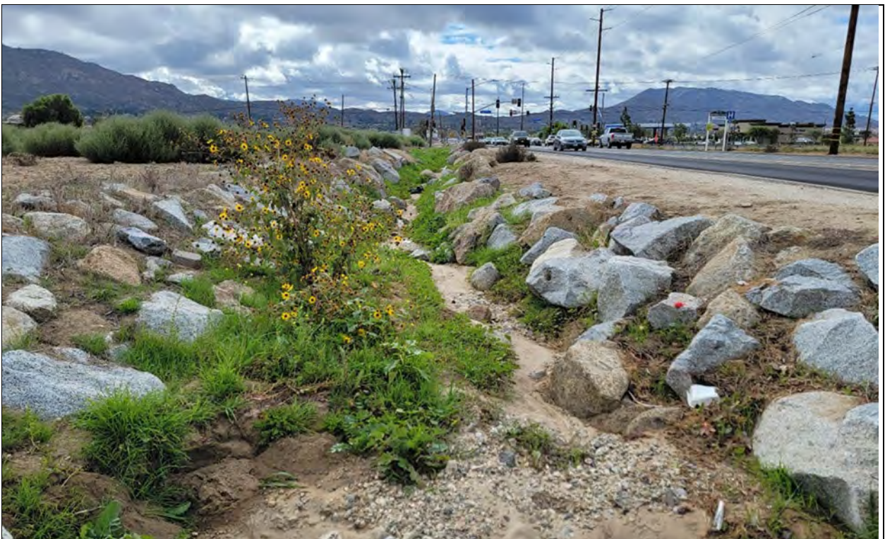
Photograph 18: View of Drainage 4 facing downstream and south, north of Alessandro Boulevard where Drainage 4 continues as an ungrouted rip rap channel.
