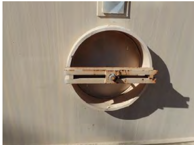
Figure 19: Manway entrance in good condition and mild corrosion on cross member and bolt
